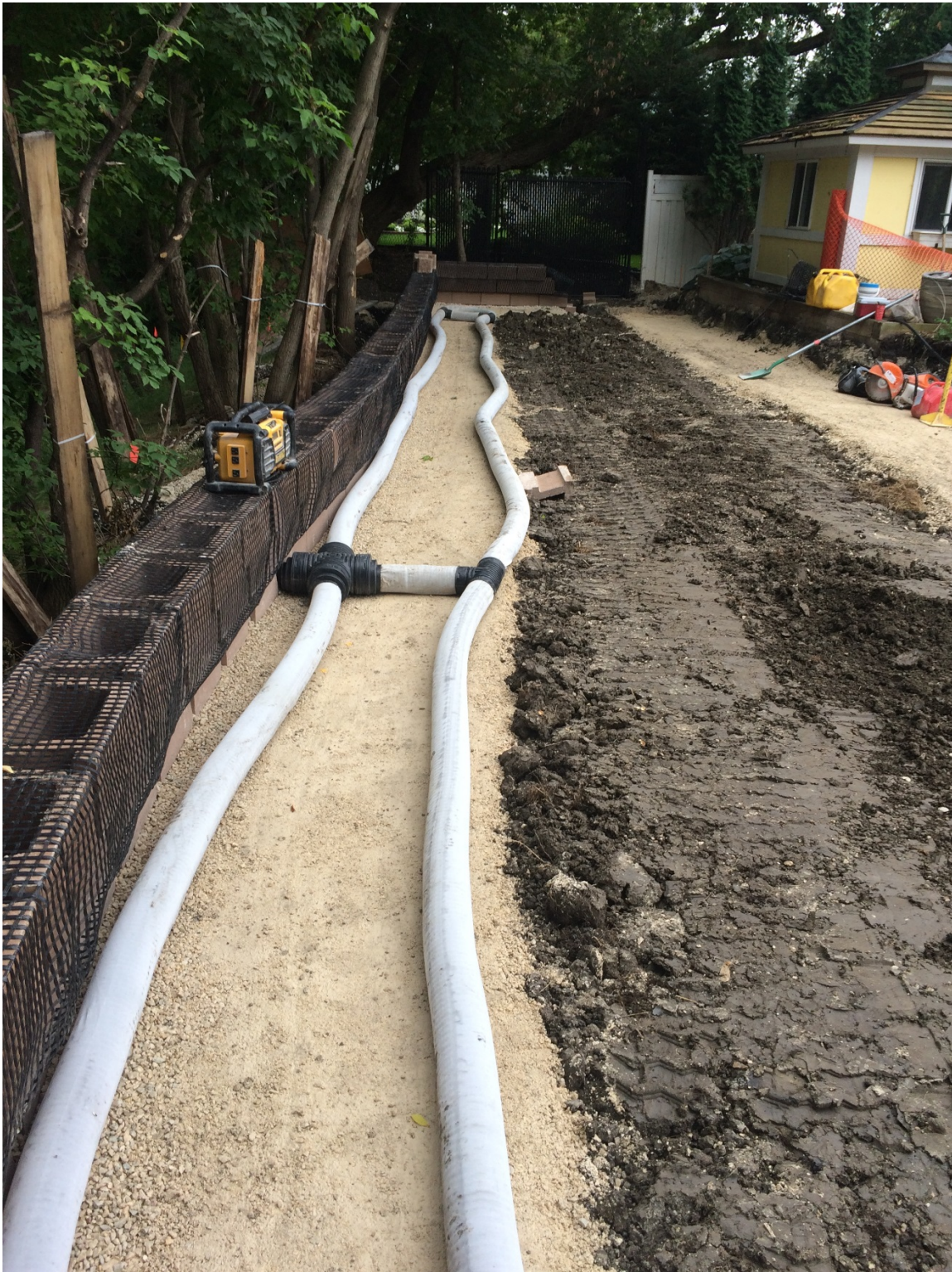
Photo 2 - Placement of toe and heel drains behind creek side segmental block wall at 1020 Highland Park Drive.
