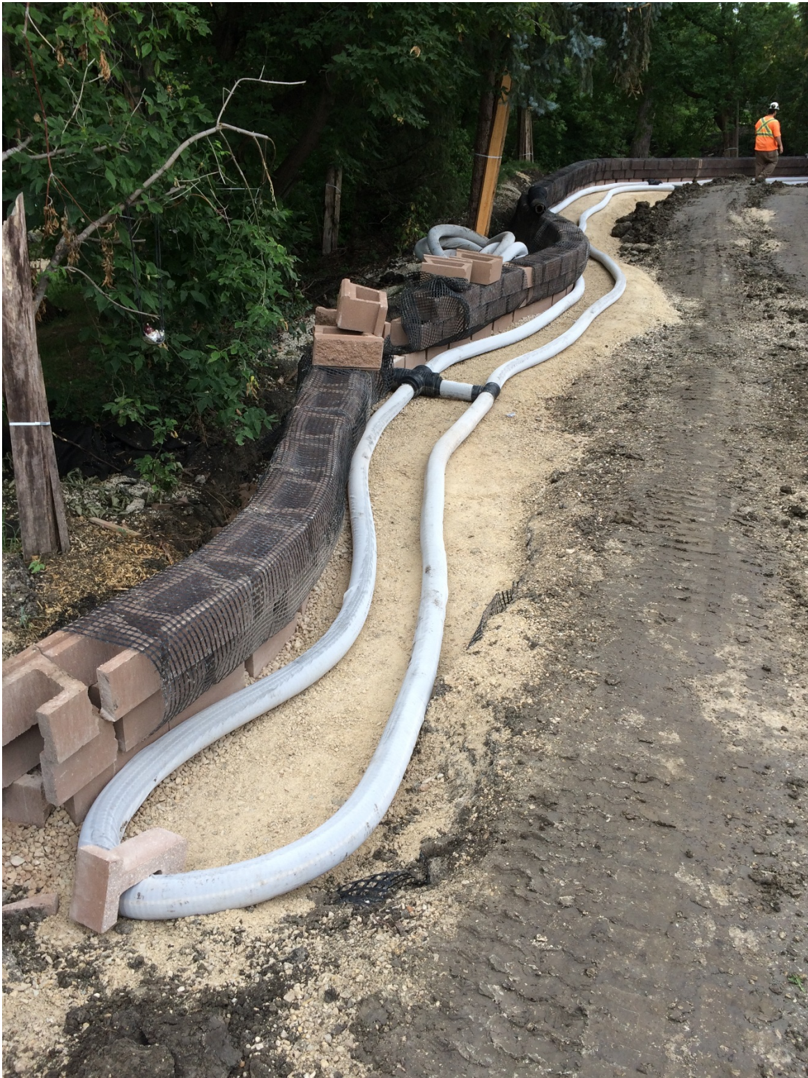
Photo 3 - Placement of toe and heel drains behind creek side segmental block wall at 1030 Highland Park Drive.
