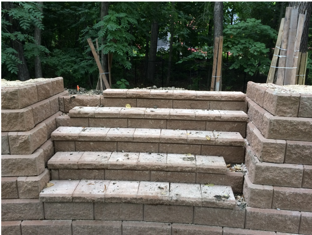
Photo 1 - Start of stair placement in creek side segmental block wall at 3154 Henderson Highway.
