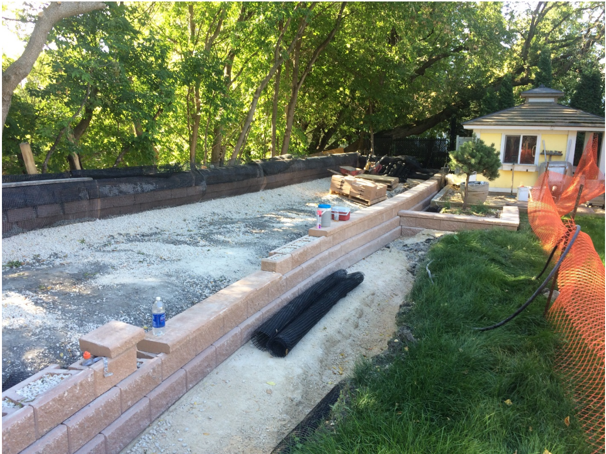
Photo 5 - Stair location on lower terrace segmental block wall at 1020 Highland Park Drive.
