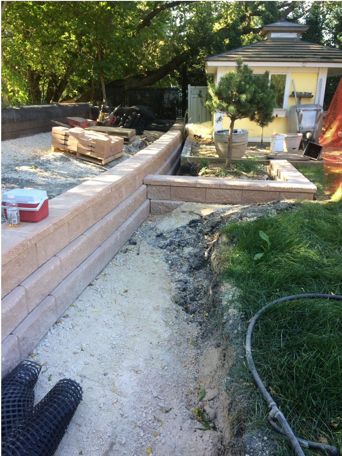
Photo 4 - Lower terrace segmental block wall placed on house side of the new dike and blocks placed around the tree at 1020 Highland Park Drive.
