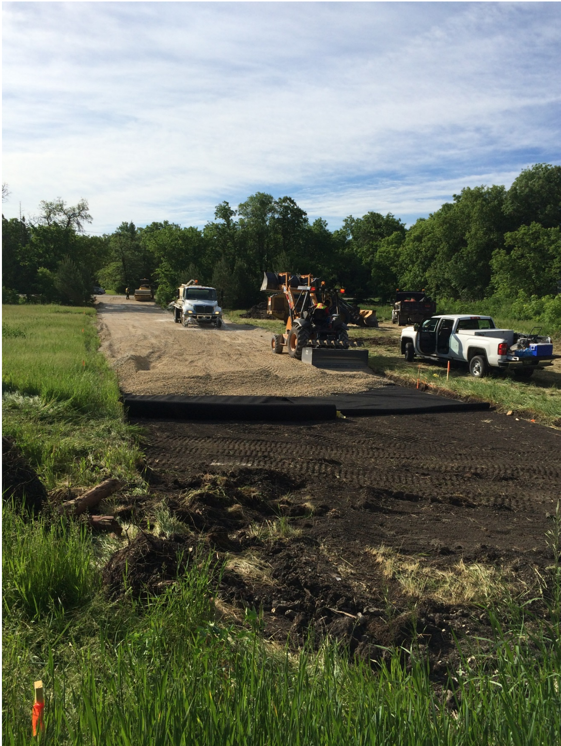
Photo 3 - Placement of geotextile and granular subbase for construction access road at 3144 Henderson Highway.
