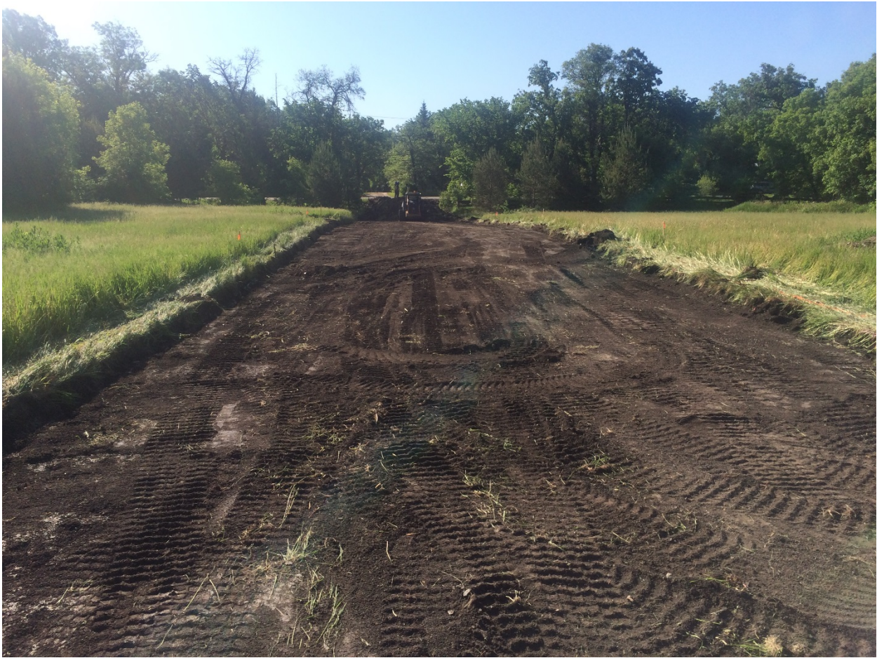
Photo 2 - Removal of organics and topsoil for placement of construction access road at 3144 Henderson Highway.
