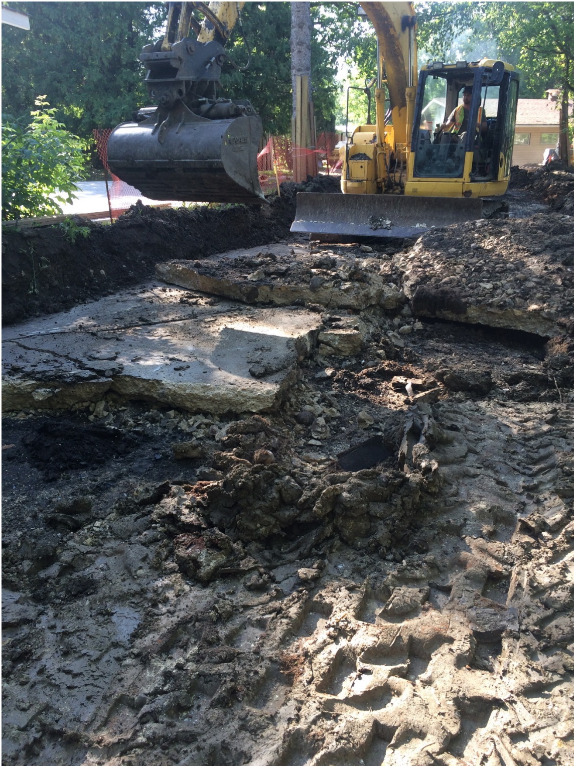
Photo 3 - Removal of the concrete garage pad below the footprint of the dike at 3144 Henderson Highway.
