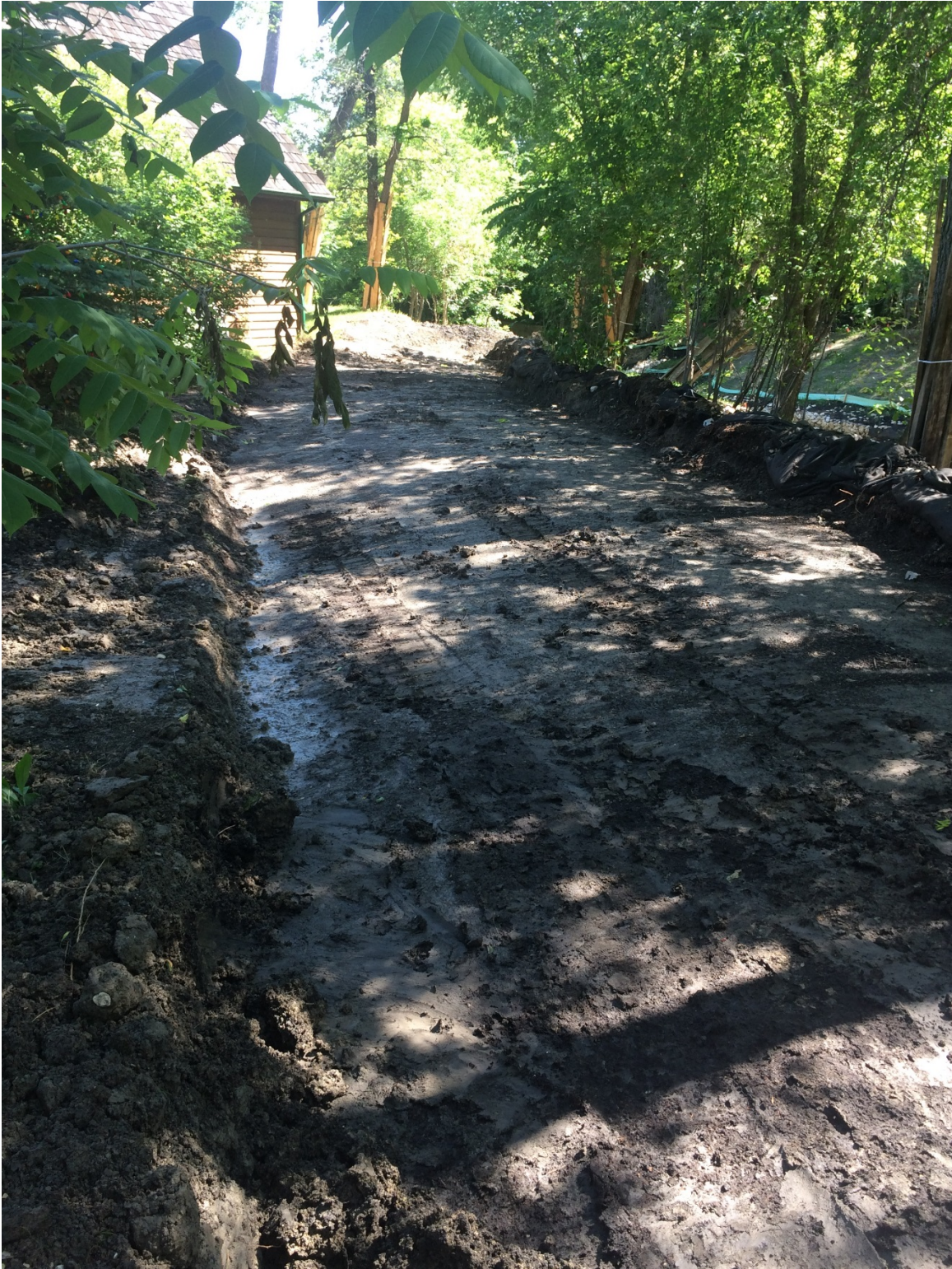
Photo 3 - Organic material removed below footprint of new dike at 1040 Highland Park Drive.
