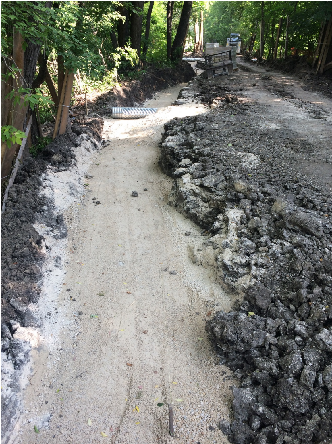
Photo 4 - Culvert installed at 3154 Henderson Highway and foundation for segmental block wall completed.
