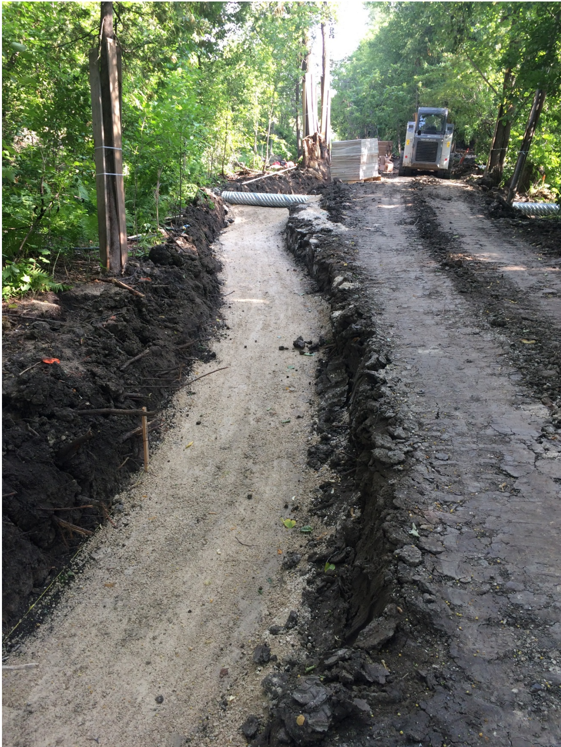
Photo 5 - Culvert installed at 3154 Henderson Highway and foundation for segmental block wall completed.
