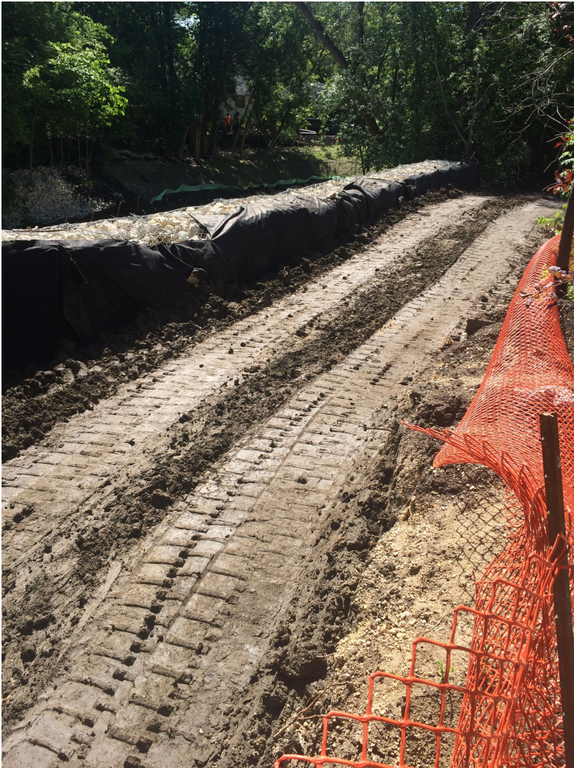
Photo 2 - Clay fill placed for new dike behind gabion baskets at 1030 Highland Park Drive.
