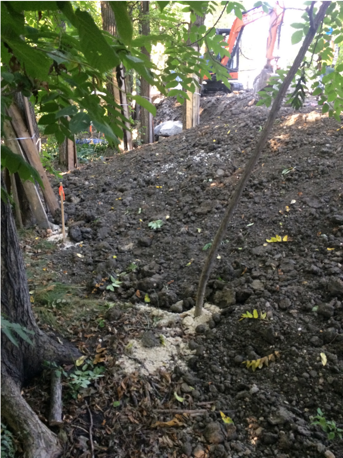
Photo 8 - Placement of clay fill for new dike side slope at 3154 Henderson Highway.
