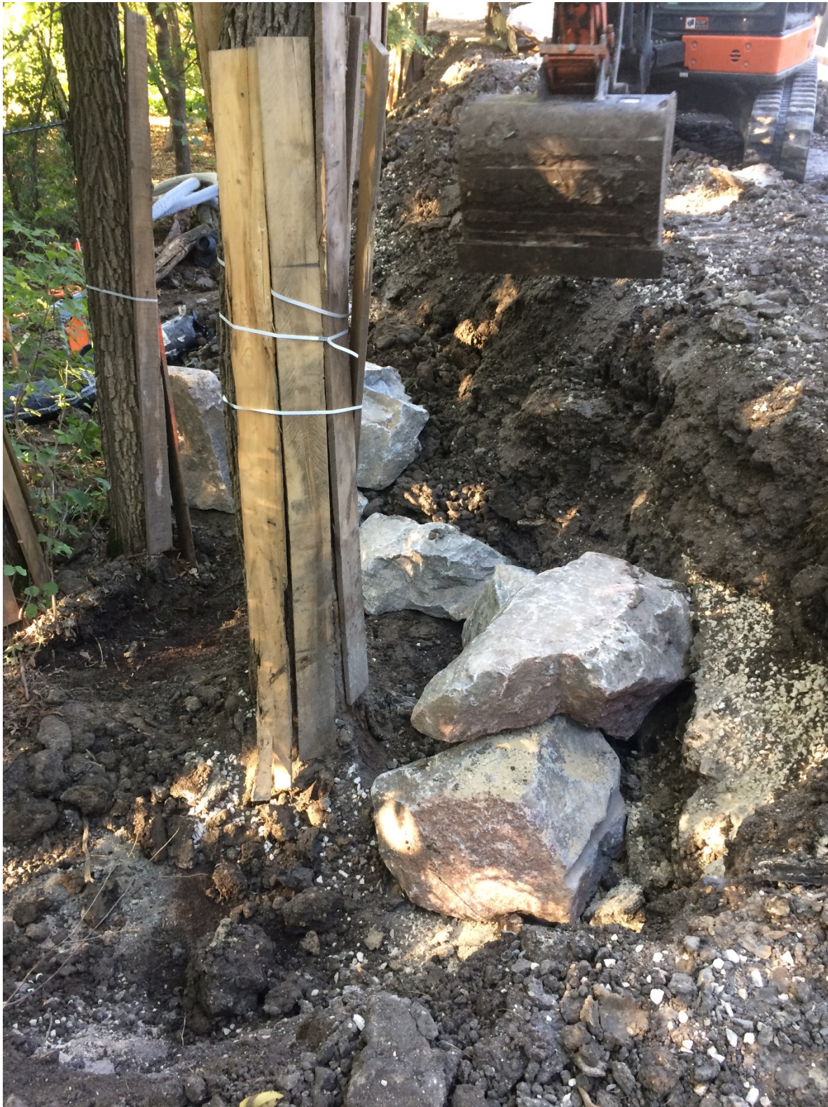
Photo 6 - Placement of clay fill for new dike and rock for tree wells at 3154 Henderson Highway.
