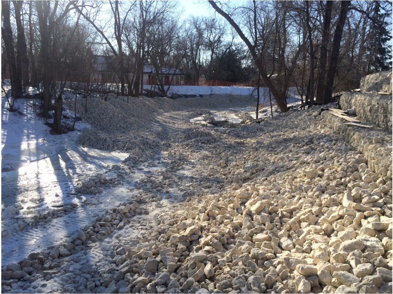
Photo 2 - Shaped rockfill toe berm at 1030 Highland Park Drive and placed rockfill at 3144 Henderson Highway.
