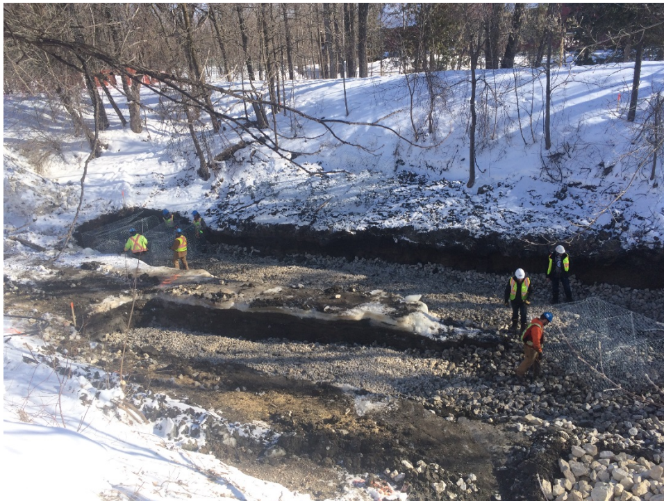
Photo 1 - Completed shear keys and gabion placement at 1040 Highland Park Drive and 3154 Henderson Highway.
