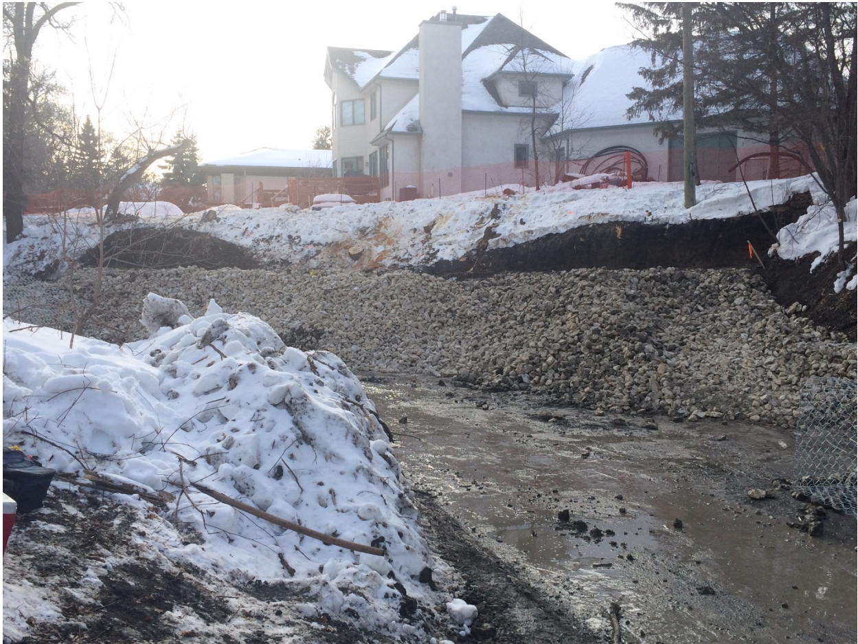
Photo 6 - Rockfill toe berm and excavated area for gabion baskets at 1030 Highland Park Drive.
