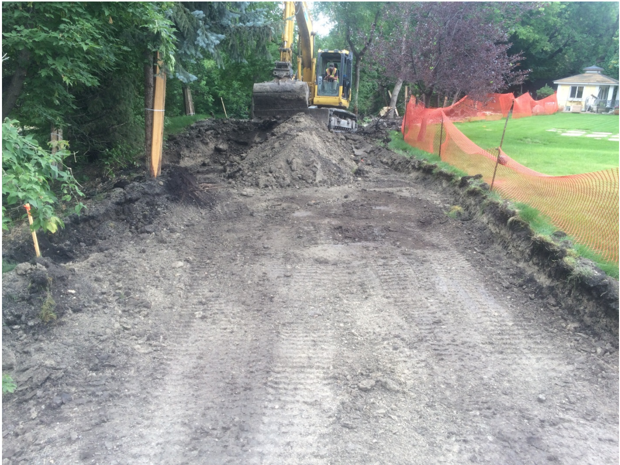
Photo 2 - Removal of organic material below footprint of new dike at 1030 Highland Park Drive.
