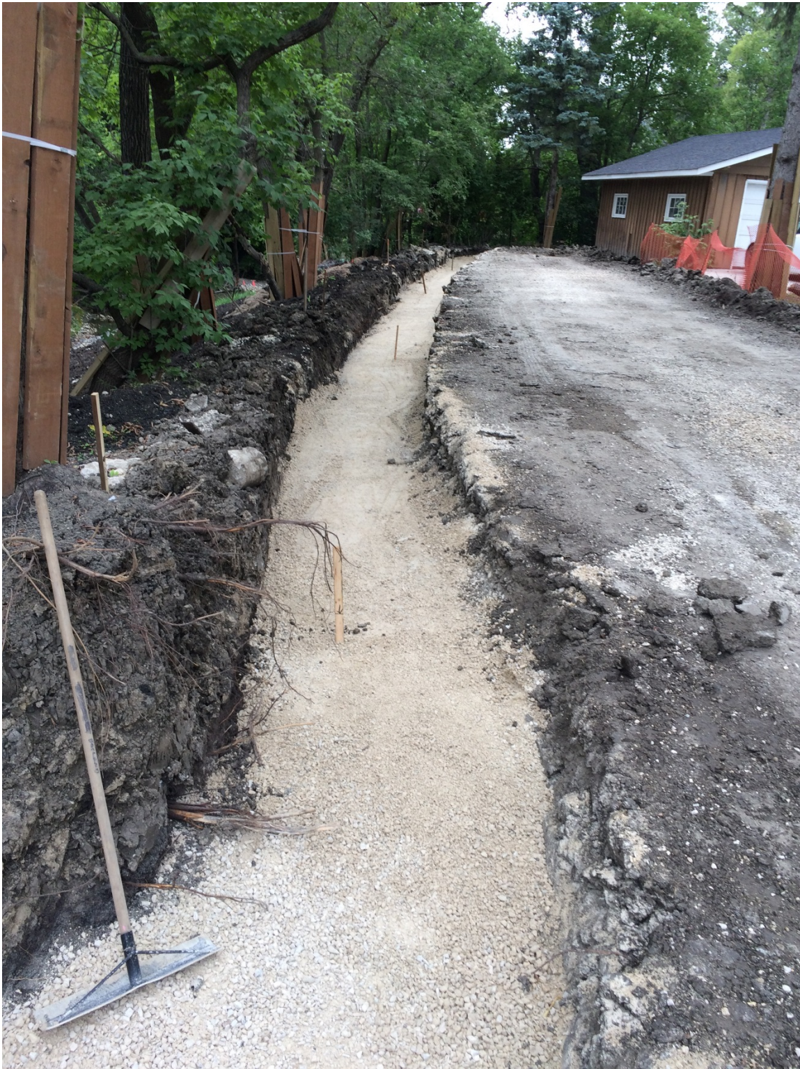
Photo 5 - Foundation for creek side segmental block wall filled with gravel at 3144 Henderson Highway.
