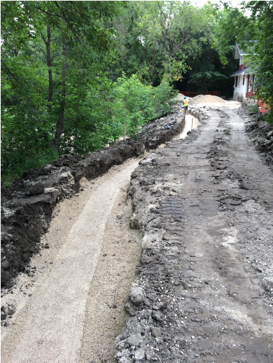
Photo 6 - Foundation for creek side segmental block wall filled with gravel at 3144 Henderson Highway.
