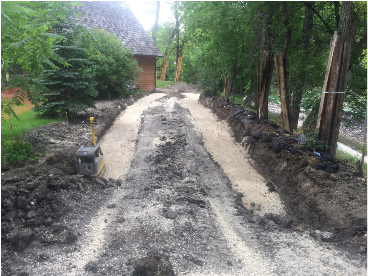
Photo 15 - Foundation for segmental block walls filled with gravel at 1040 Highland Park Drive.
