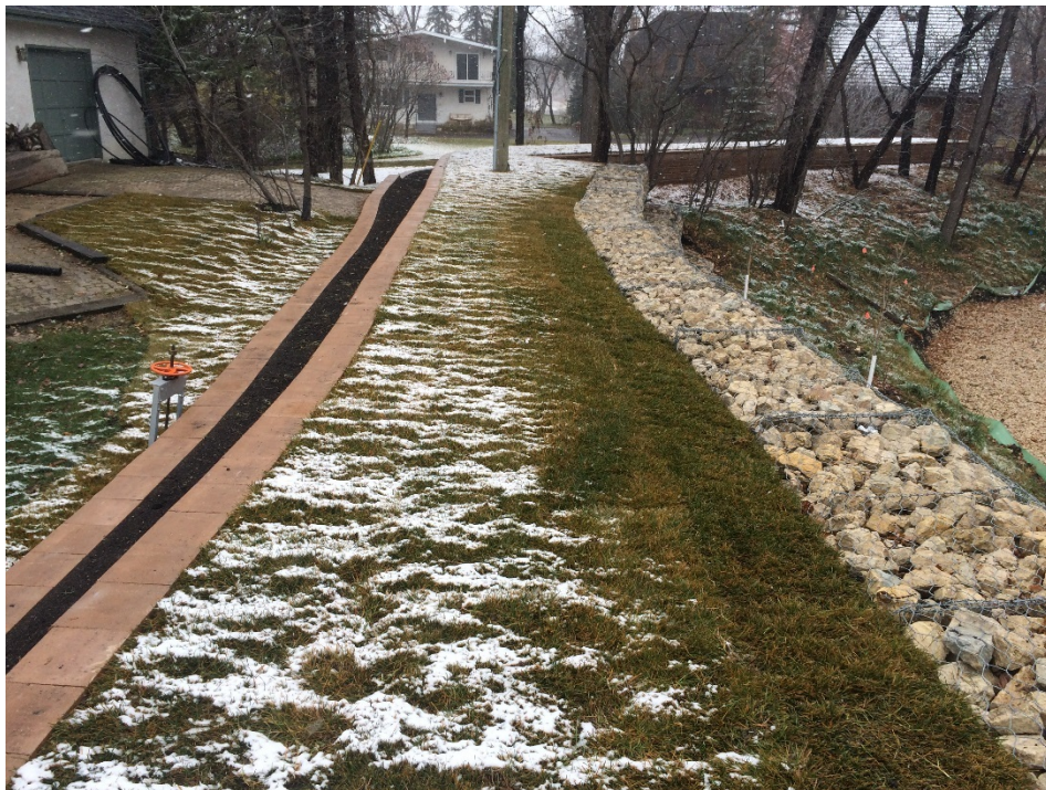
Photo 8 - Dike at 1030 Highland Park Drive.
