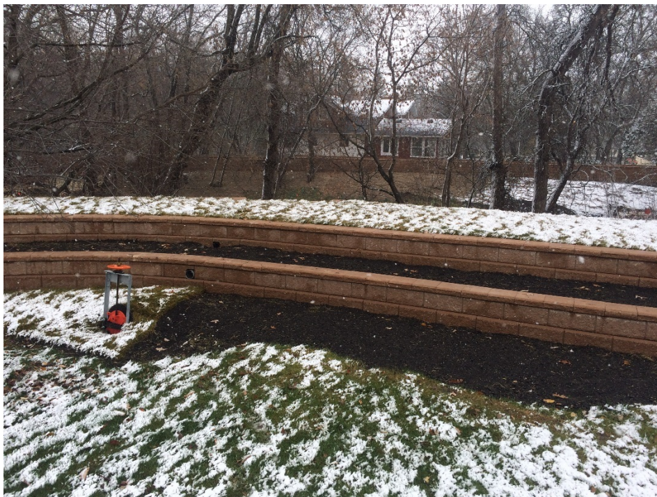
Photo 4 - Dike at 1020/1030 Highland Park Drive.
