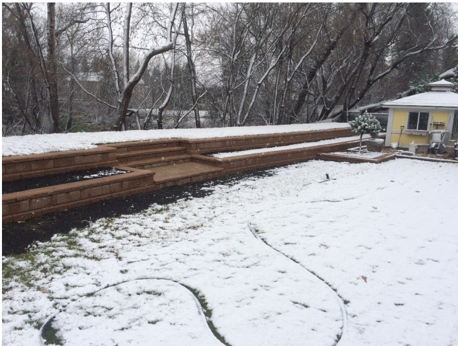
Photo 2 - Dike at 1020 Highland Park Drive.
