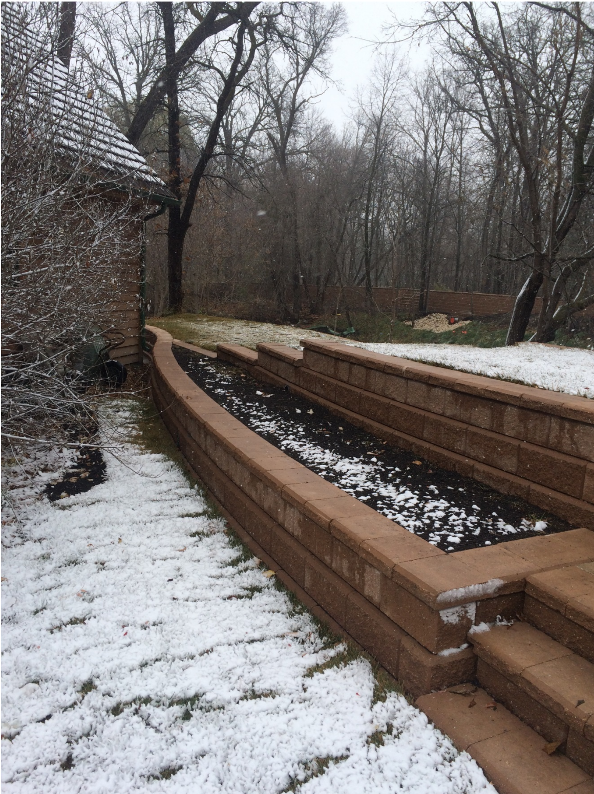
Photo 11 - Dike at 1040 Highland Park Drive.
