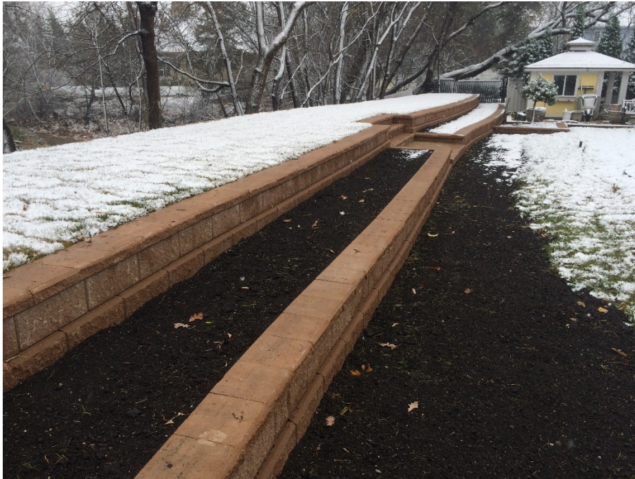
Photo 1 - Dike at 1020 Highland Park Drive.
