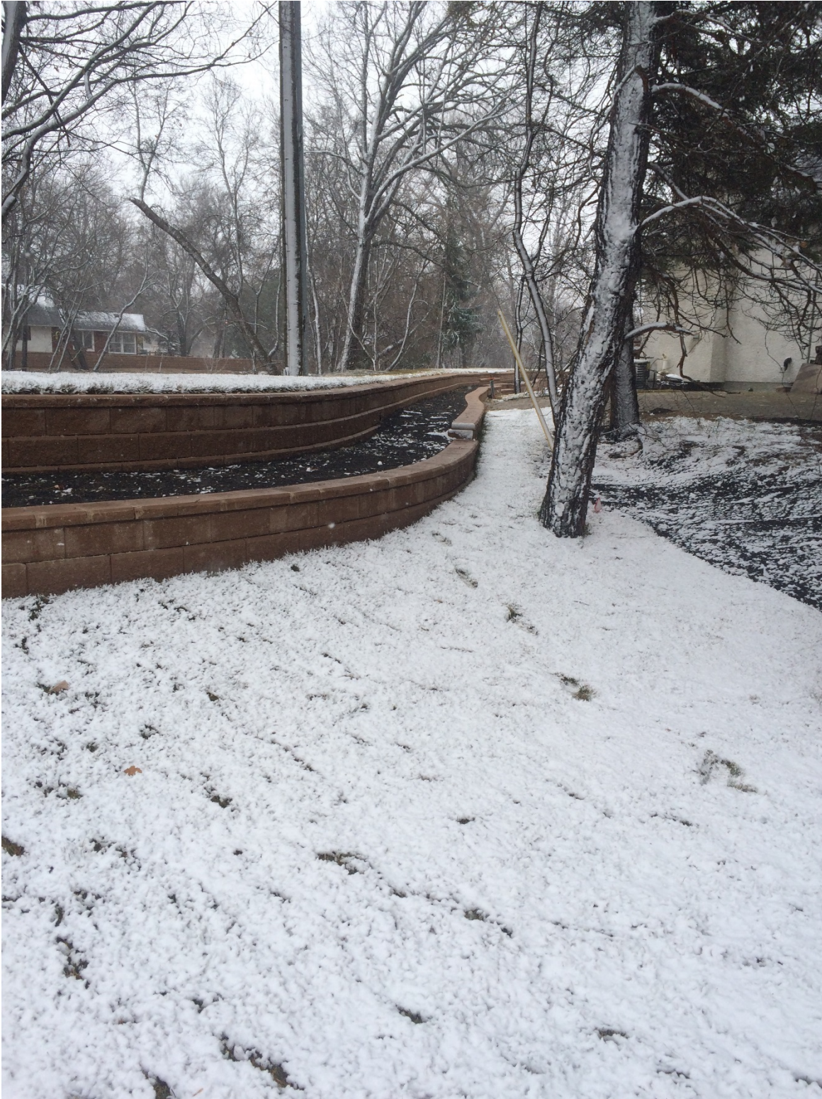
Photo 9 - Dike at 1030/1040 Highland Park Drive.
