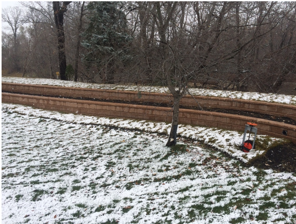
Photo 3 - Dike at 1030 Highland Park Drive.
