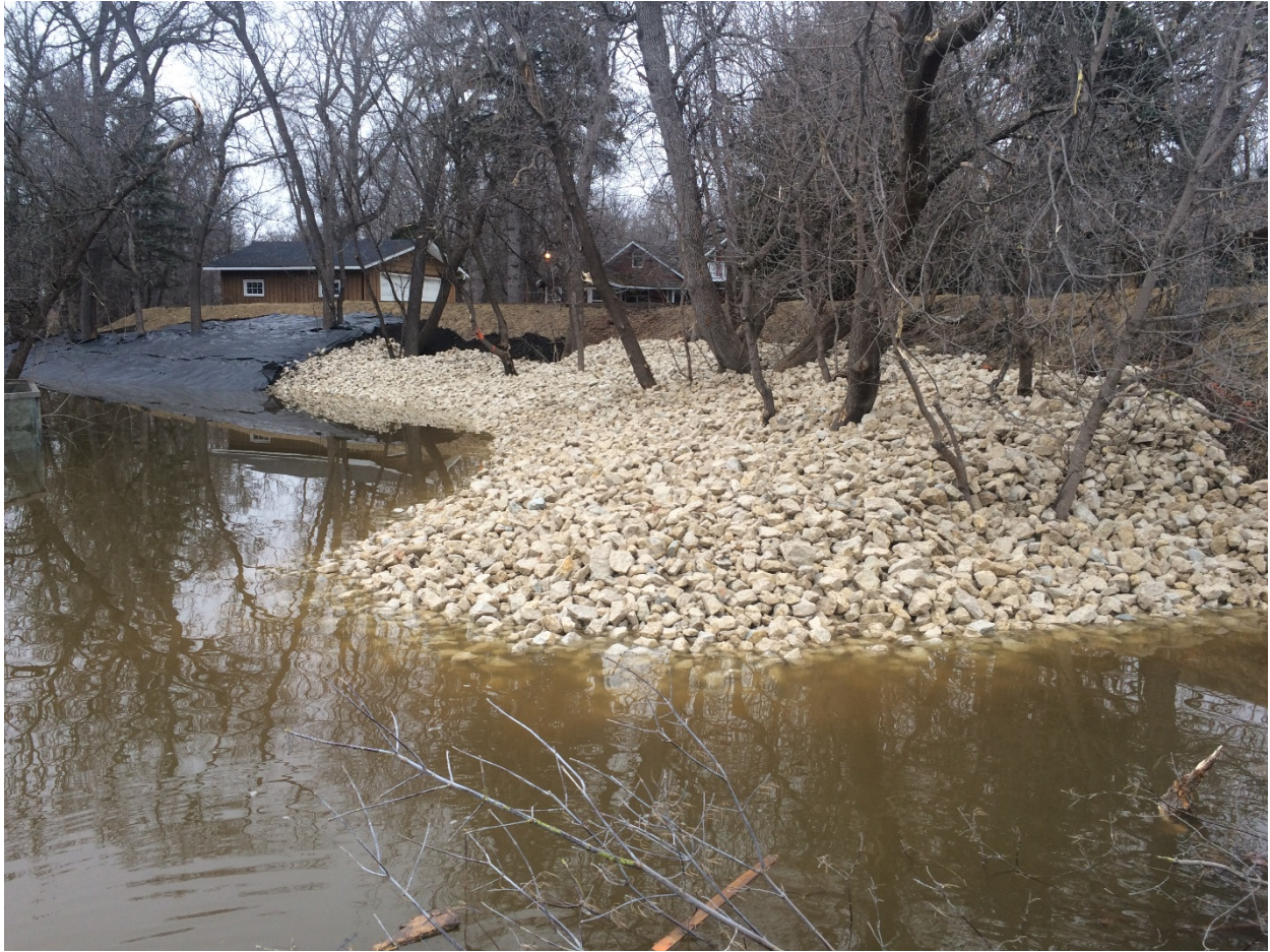
Photo 5 - Completed rockfill toe berm at 3144 Henderson Highway. Additional topsoil to be placed during Phase 2 of the project.
