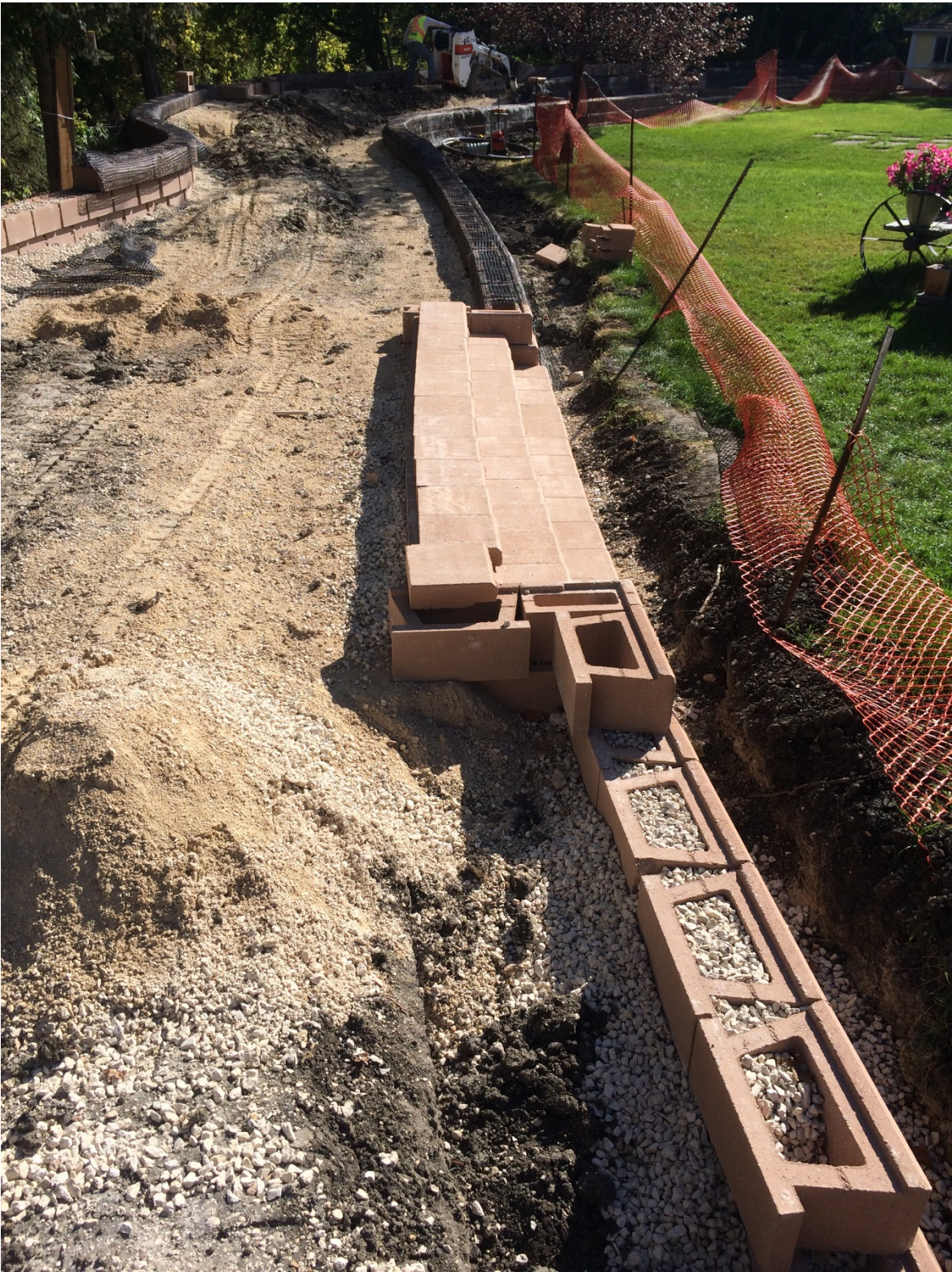
Photo 5 - Stair location on lower terrace segmental block wall at 1020 Highland Park Drive.
