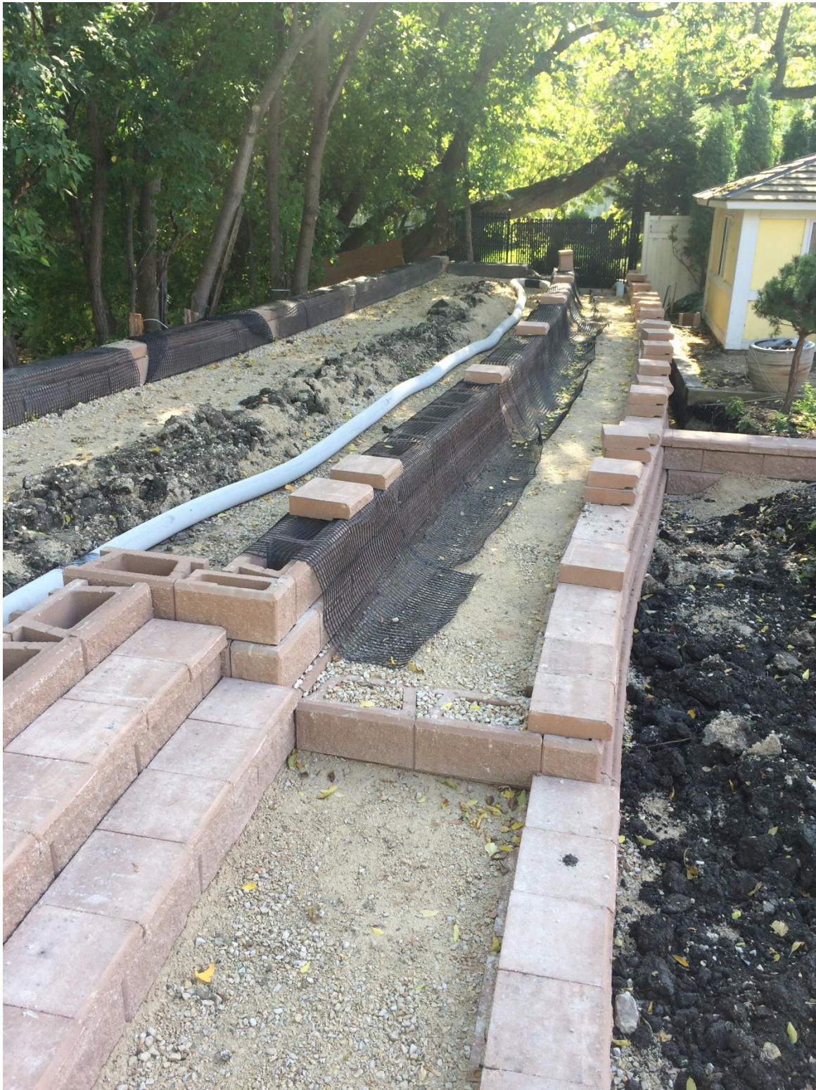
Photo 6 - Upper terrace house side segmental block wall placed at 1020 Highland Park Drive.
