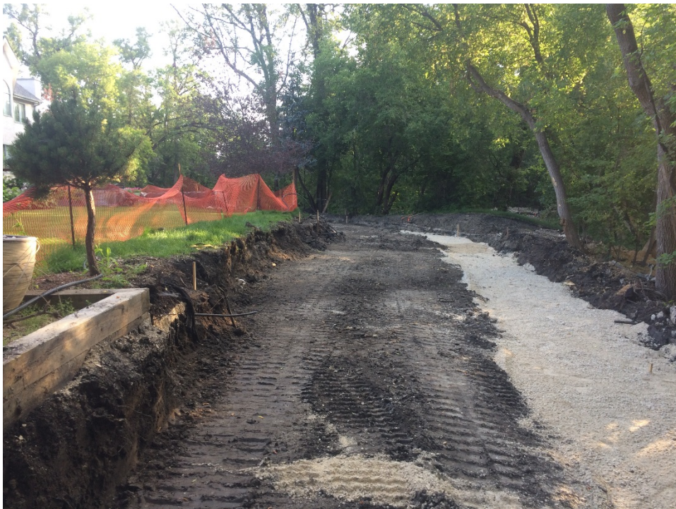
Photo 8 - Gravel placed for foundation of segmental block wall at 1020 Highland Park Drive.
