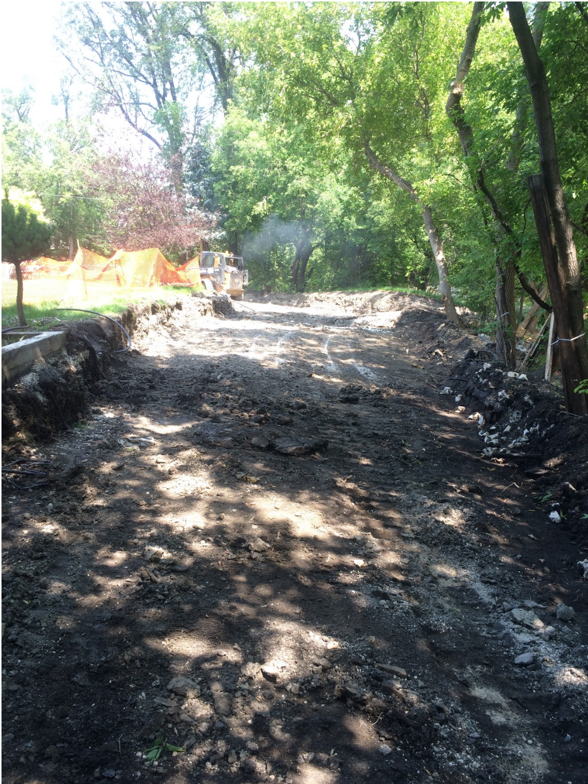
Photo 2 - Removal of organic material below footprint of new dike at 1020 Highland Park Drive.
