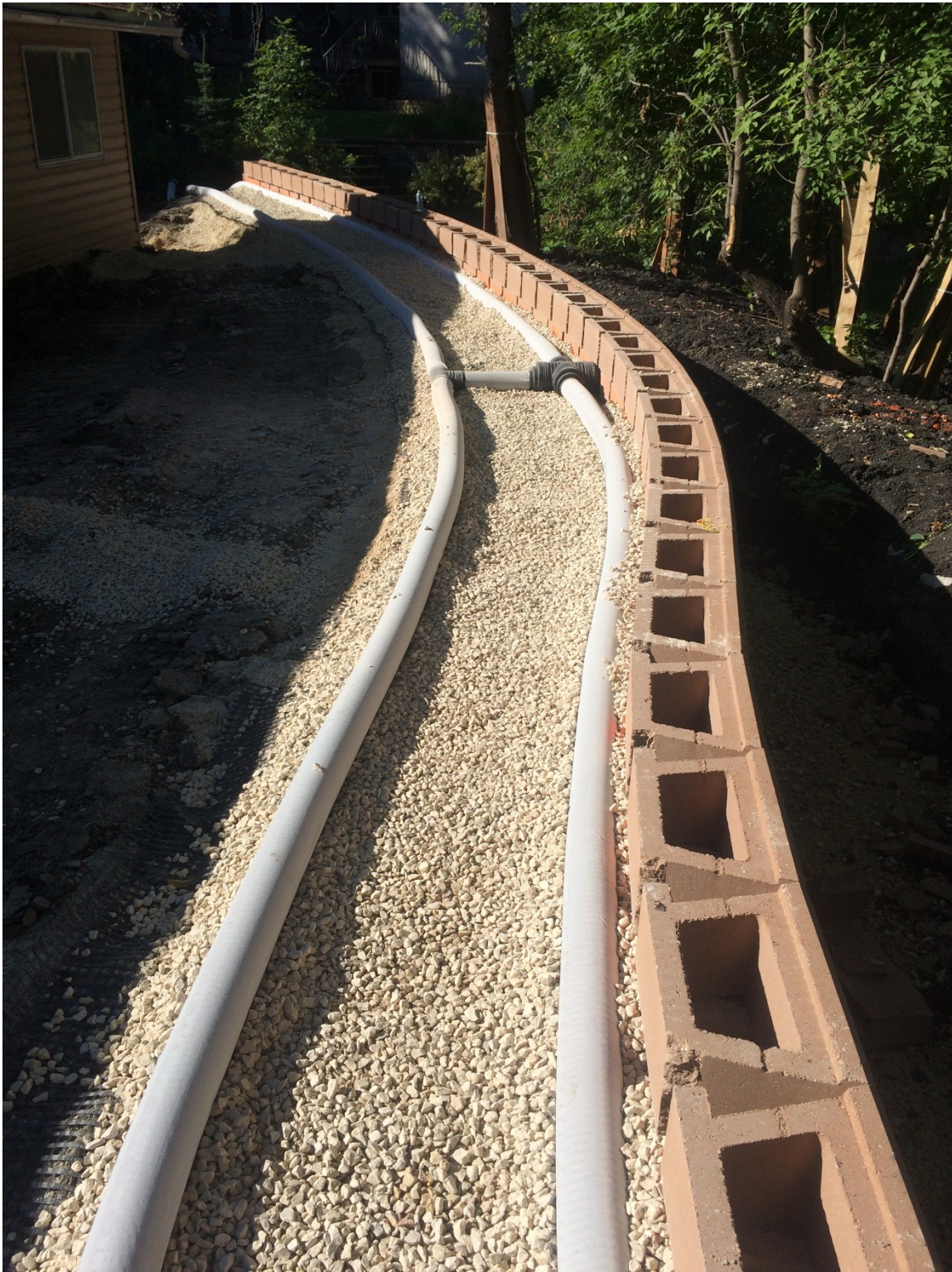
Photo 16 - Toe and heel drain installation behind creek side segmental block wall at 3144 Henderson Highway.
