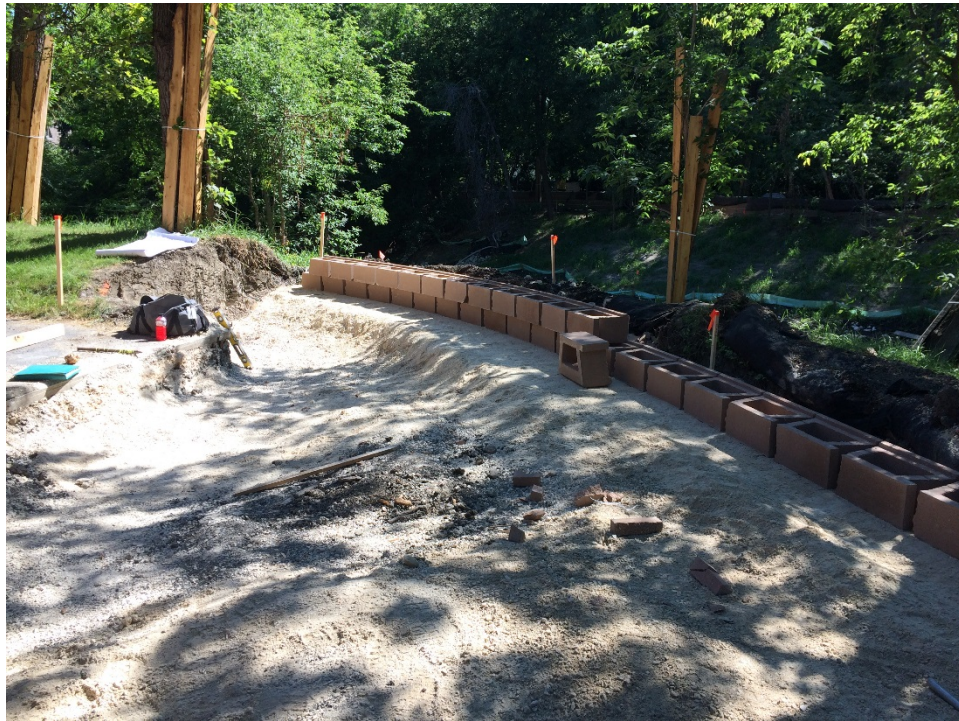
Photo 13 - Placement of the creek side segmental block wall at 1040 highland Park Drive.
