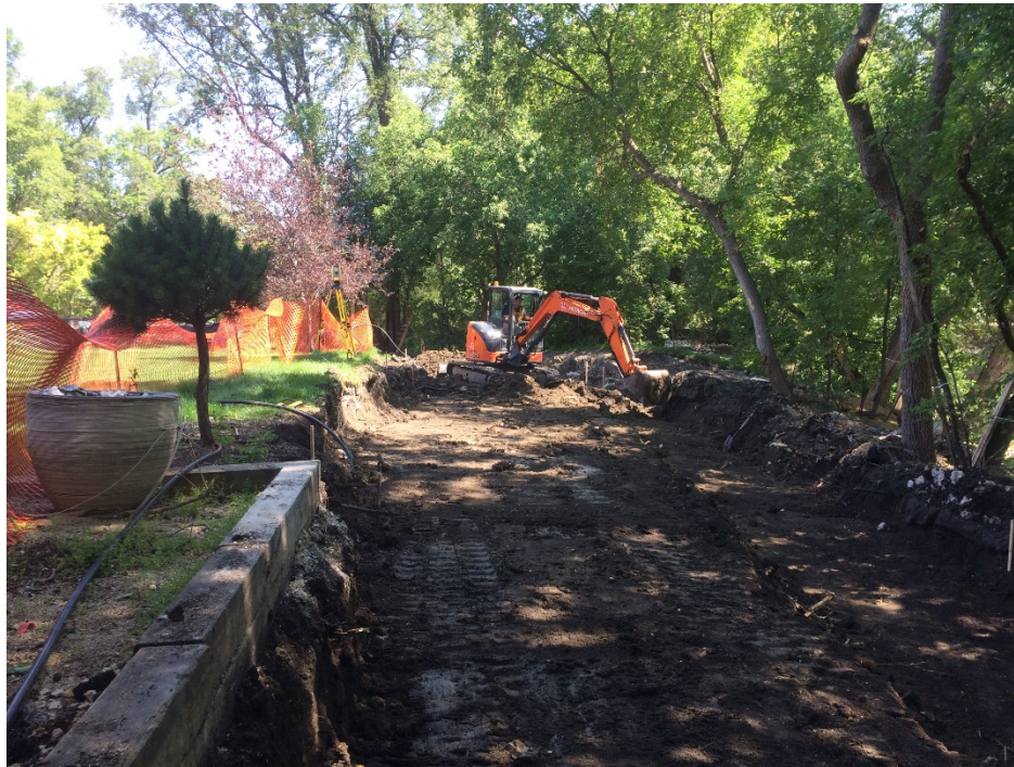
Photo 5 - Foundation for creek side segmental block wall excavated at 1020 Highland Park Drive.
