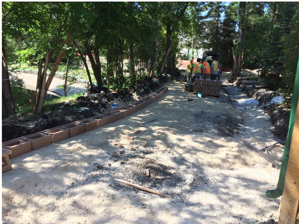
Photo 14 - Placement of the creek side segmental block wall at 1040 highland Park Drive.
