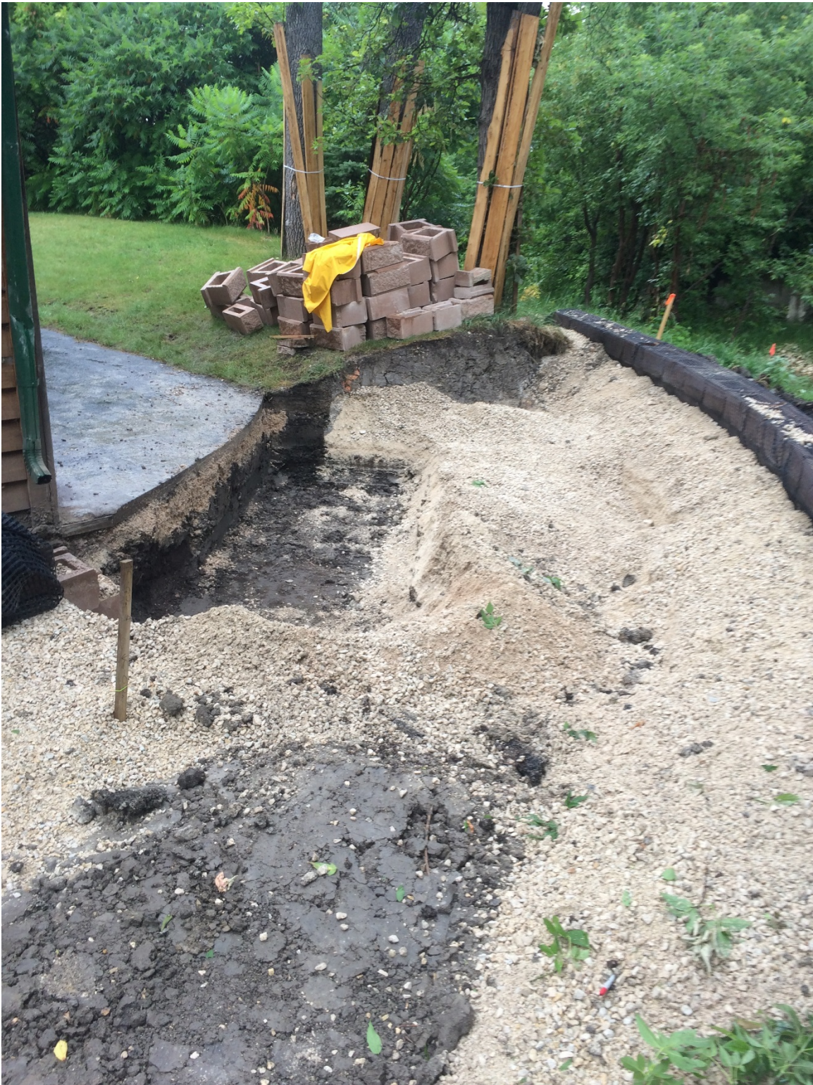
Photo 20 - Removal of asphalt driveway for house side segmental block wall placement at 1040 Highland Park Drive.
