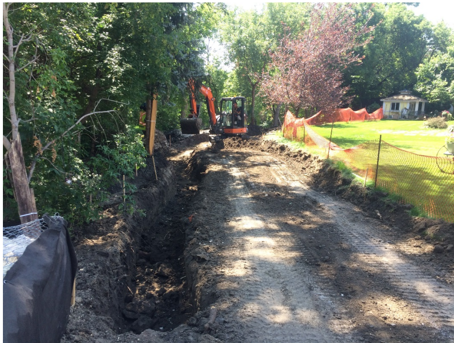
Photo 6 - Foundation for creek side segmental block wall excavated at 1030 Highland Park Drive.
