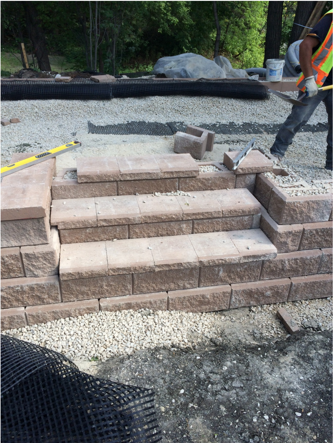
Photo 23 - Stair construction on house side segmental block wall at 1040 Highland Park Drive.
