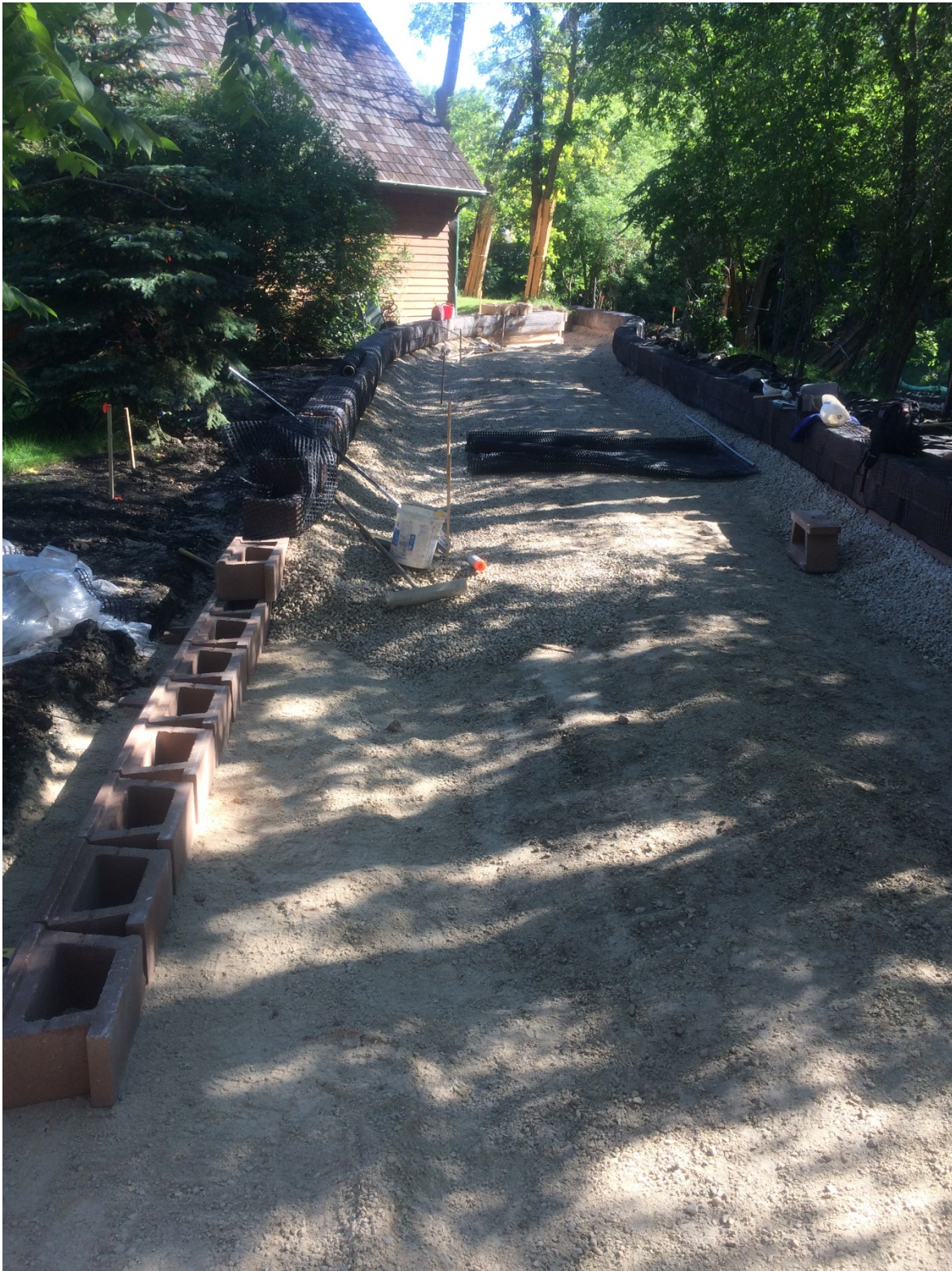
Photo 15 - Placement of the house side segmental block wall at 1040 Highland Park Drive.
