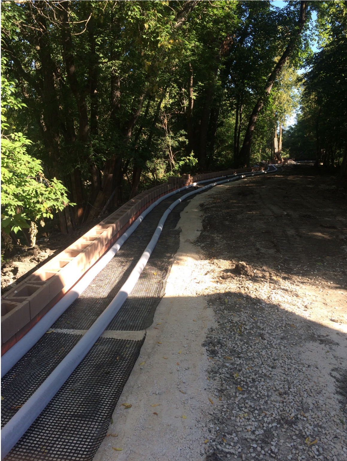
Photo 17 - Toe and heel drain installation behind creek side segmental block wall at 3144 Henderson Highway.
